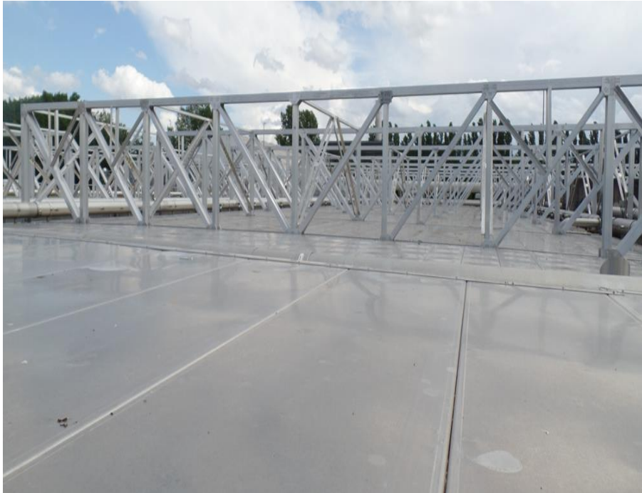
Biological Aeration Basins Coverage for aeration tanks
