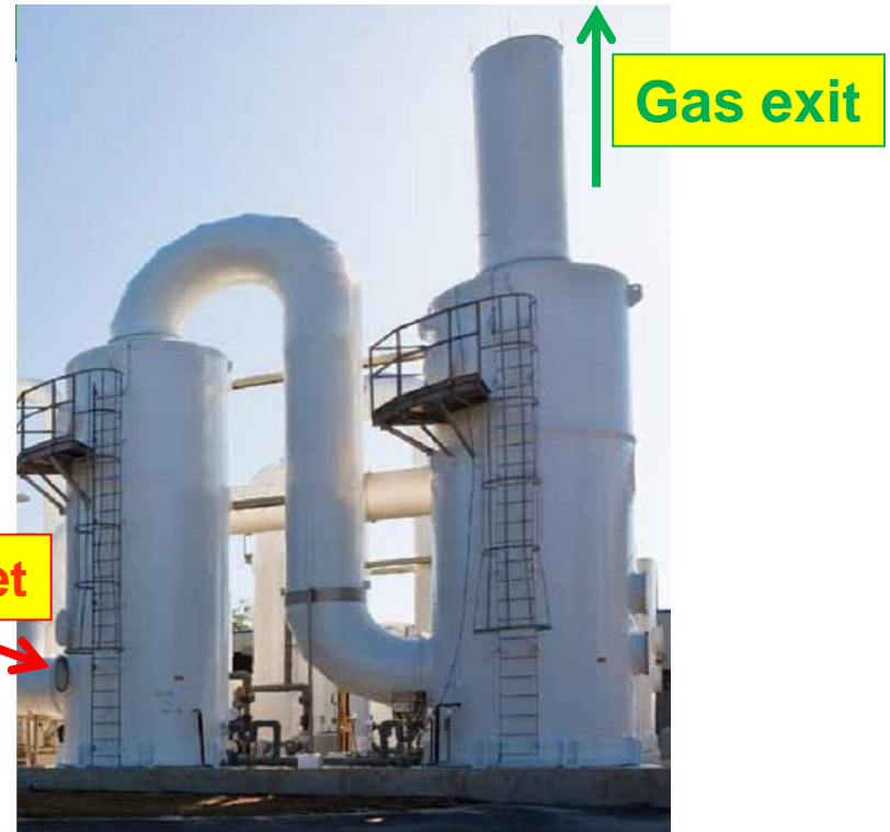
Two wet scrubbers in series
