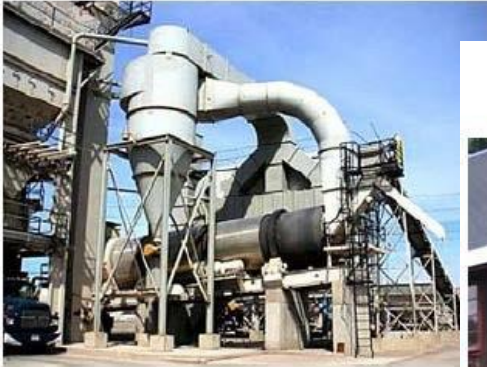
Low-pressure drop cyclone at Rochester Asphalt Plant (Victor, NY)
