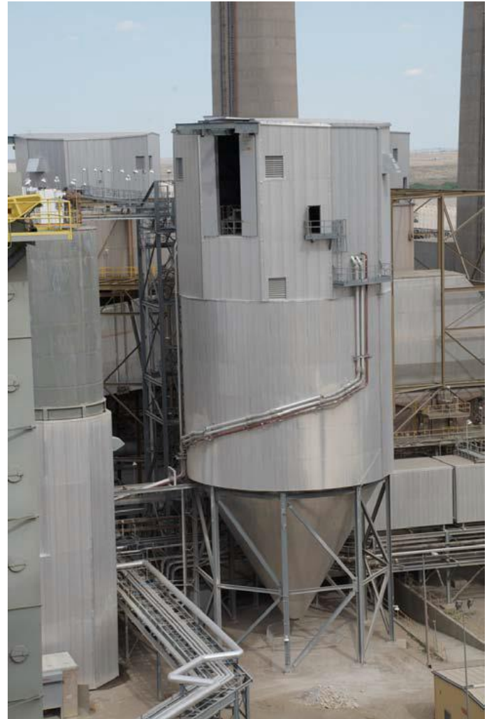
Typical dry FGD Spray Dryer Absorber
