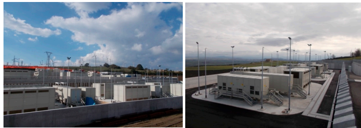
Figure 2. Some photos of Italian Na-S “energy intensive” installation in Ginestra.
