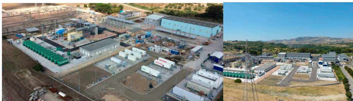
Figure 3. Two views from above the Codrongianos substation.
