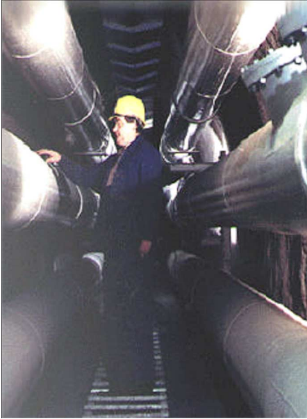
Fig. 1. Wehr (Germany) tunnel with a double-circuit GIL at 420 kV (in service since 1975, Siemens).
