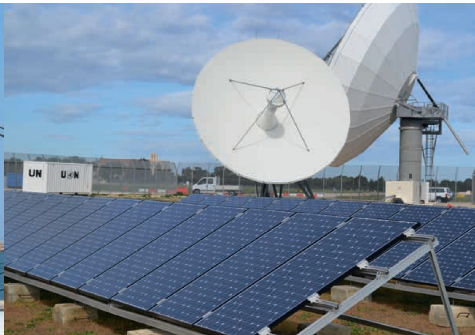
Progetto Green Island per lo UN Department of Field Support. Base logistica delle Nazioni Unite a Brindisi, luglio 2011 (Foto UNLB) Green Island Project for the UN Department of Field Support. United Nations Global Service Centre/UNLB Brindisi, July 2011 (UNLB Photo)
